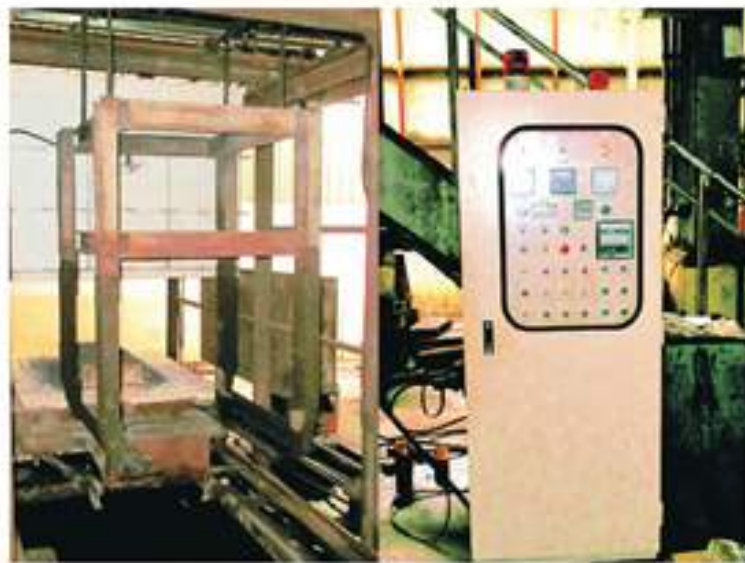
▼熱處理設備 FURNACE FOR HEAT TREATMENT
